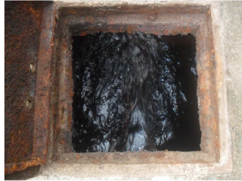
I002) Wastewater After Treatment (ETP Outlet)
